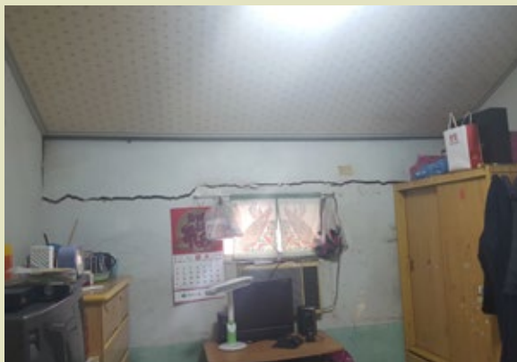
Horizontal cracks on the upper part of the wall inside the house (Before repair)
