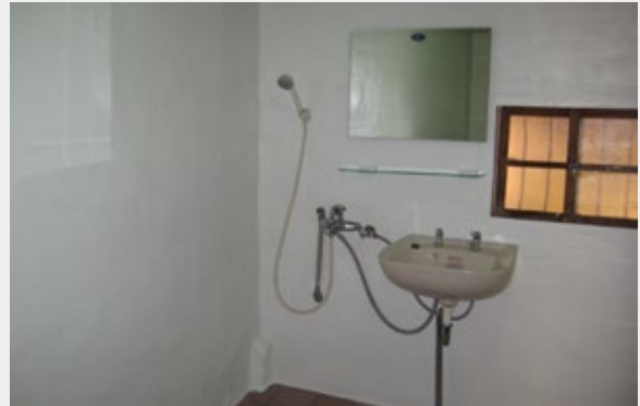
After construction, the walls in the bathroom was plastered and repainted, and a sink and a mirror were installed
