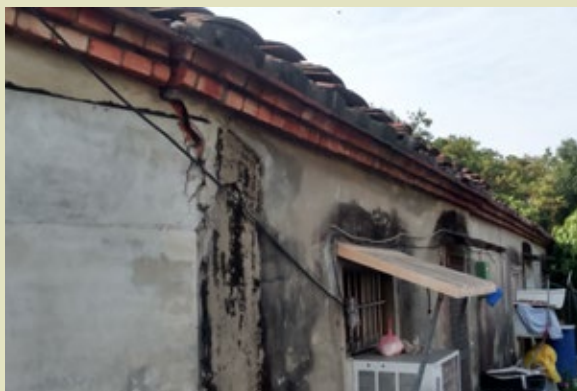
Horizontal cracks on the top of the external brick wall and bulging walls (Before repair)
