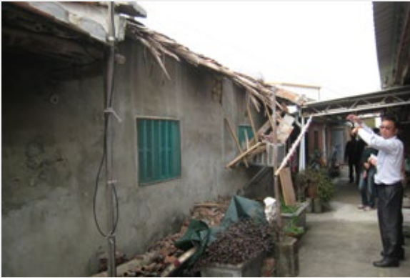
The damaged rooftop (before repair)
