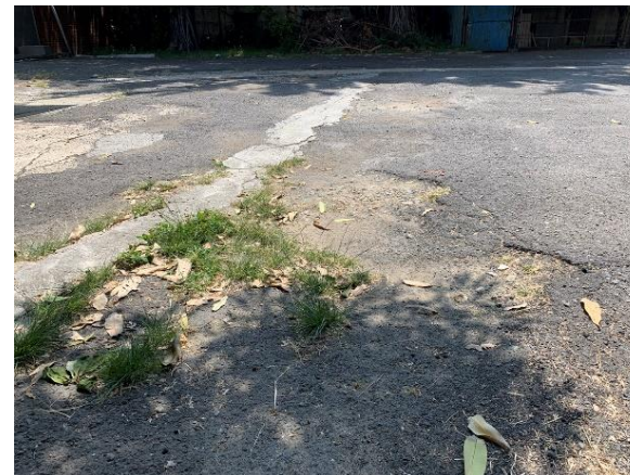
樹木竄根，柏油破損
