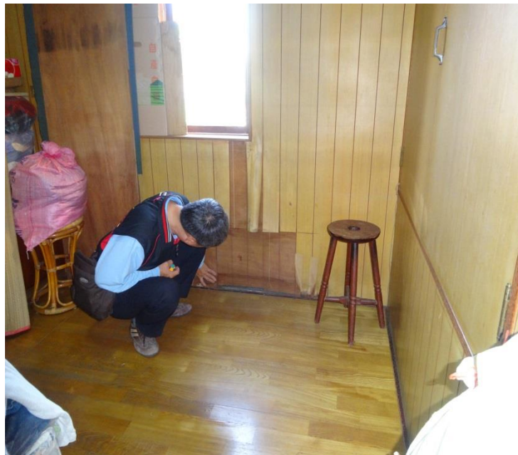
牆壁木板掀起
